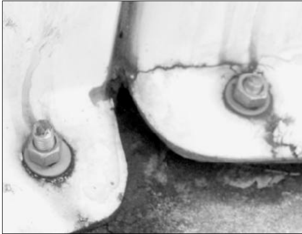
Pictured above is at least one crack that has formed in the temporary jail facility at the county courthouse. (Staff photo by Stephen Crews)
